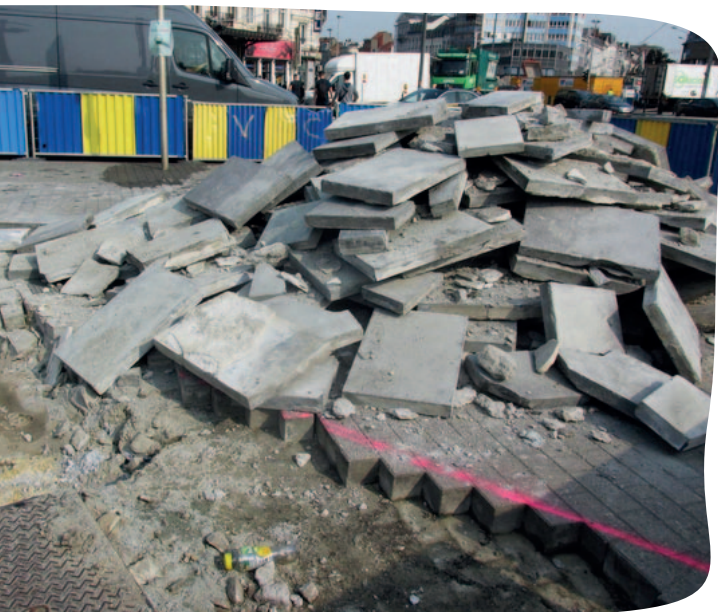
Road construction site in Brussels, September 2020. Blue stone floor slabs are dismantled without particular care: through this action, the contractor discards the materials and legally transforms them into waste.
