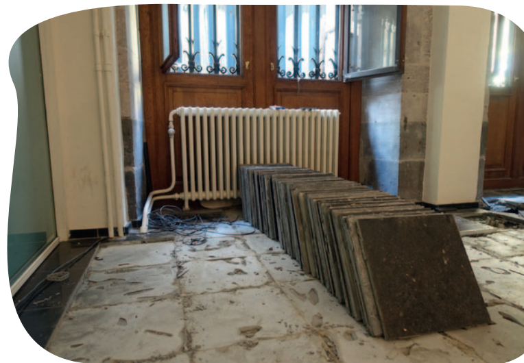
Dismantling natural stone slabs, Antwerp 2018. The slabs have been identified in an inventory of potential materials for reuse in a public building. They are the subject of targeted removal by a specialised operator, who will also ensure their resale in a well-established market. The panel of indicators clearly converges on the side of a classification as a ‘product’.
